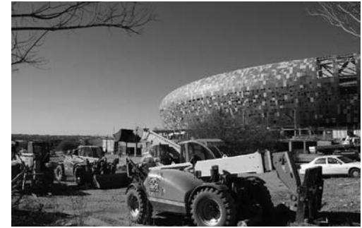
Interrupted construction works Workers on strike at different stages of the building of stadia that hosted the World Cup (Larger photo: Warrenski/CC; photo above: Shine/CC)
